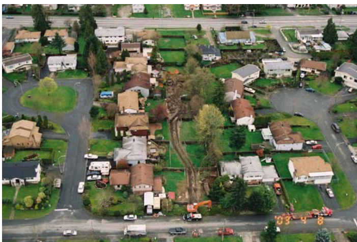
Precise cadastral data helps to ensure the accuracy of digs in urban areas.
