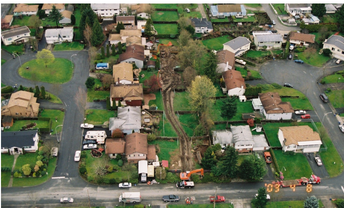
Precise cadastral data helps to ensure the accuracy of digs in urban areas.
